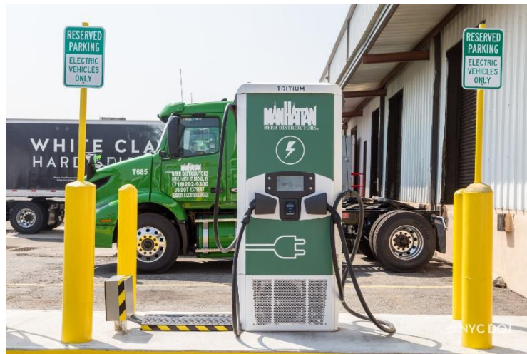
An electric truck charger at Manhattan Beer Bronx facility
