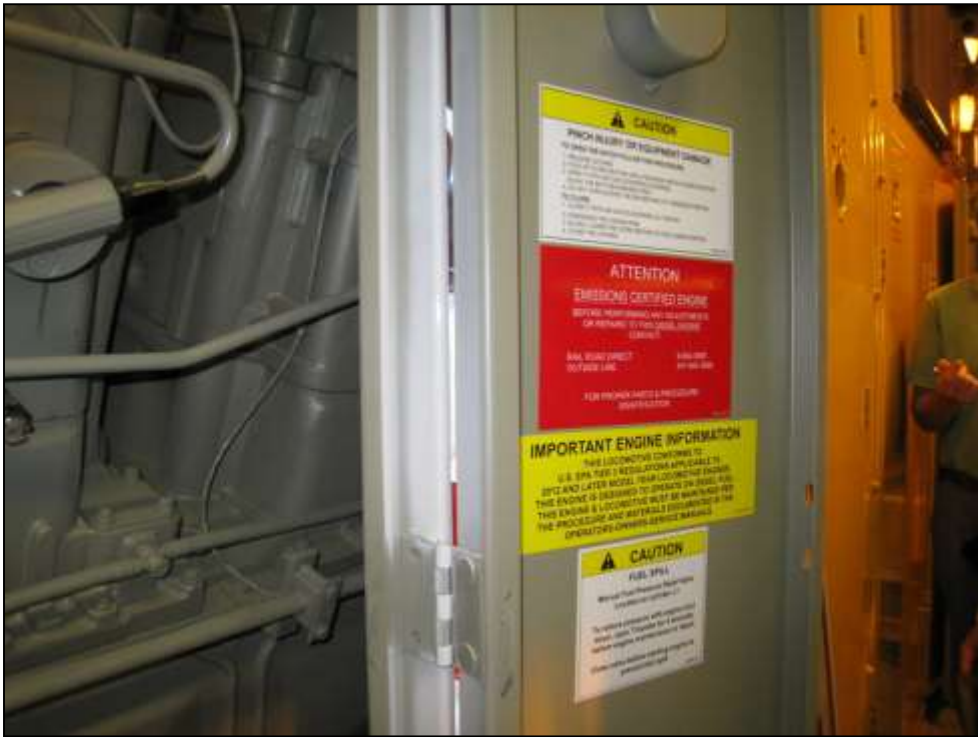
Supplemental labels on the engine cabinet door.
